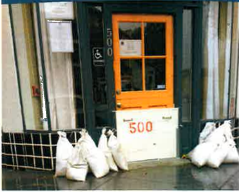
Neighbors prepare for stormy weather by protecting doorways with sandbags and floodgates.
