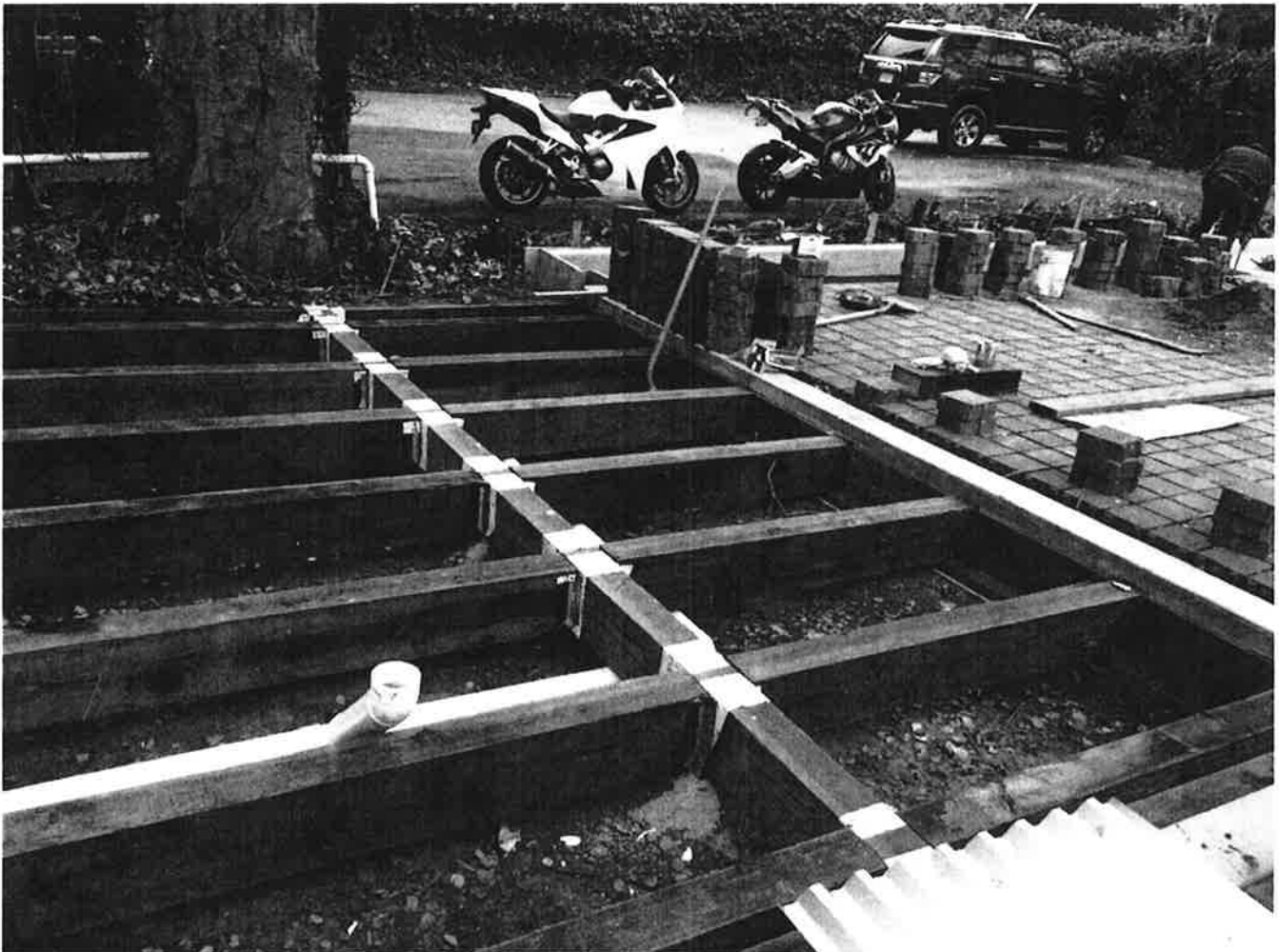
Figure 1. Raised parking deck with perforated pipe running beneath to disperse water from drains in the deck.
