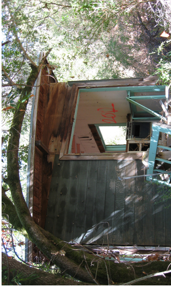
View 3. View of existing dilapidated cabin on-site.
