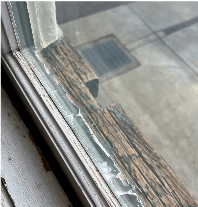
Public Safety Building - Deteriorated Window
