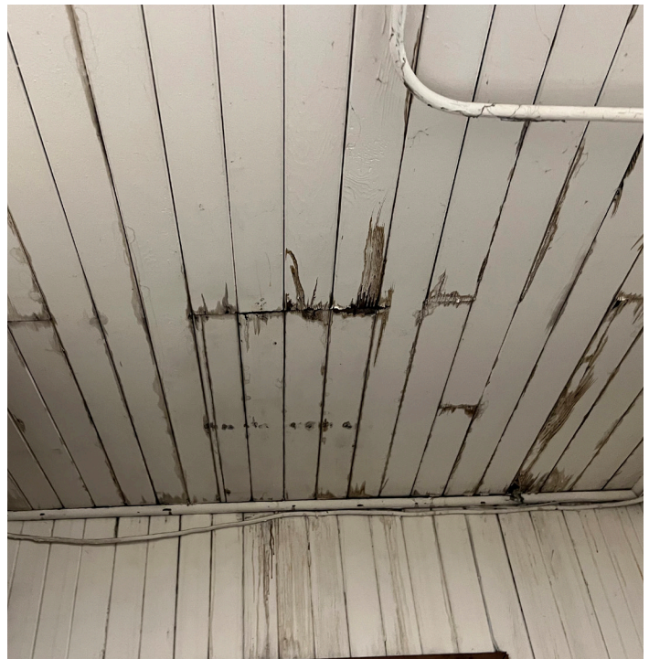
Police Department – Deteriorated Ceiling/Wall
