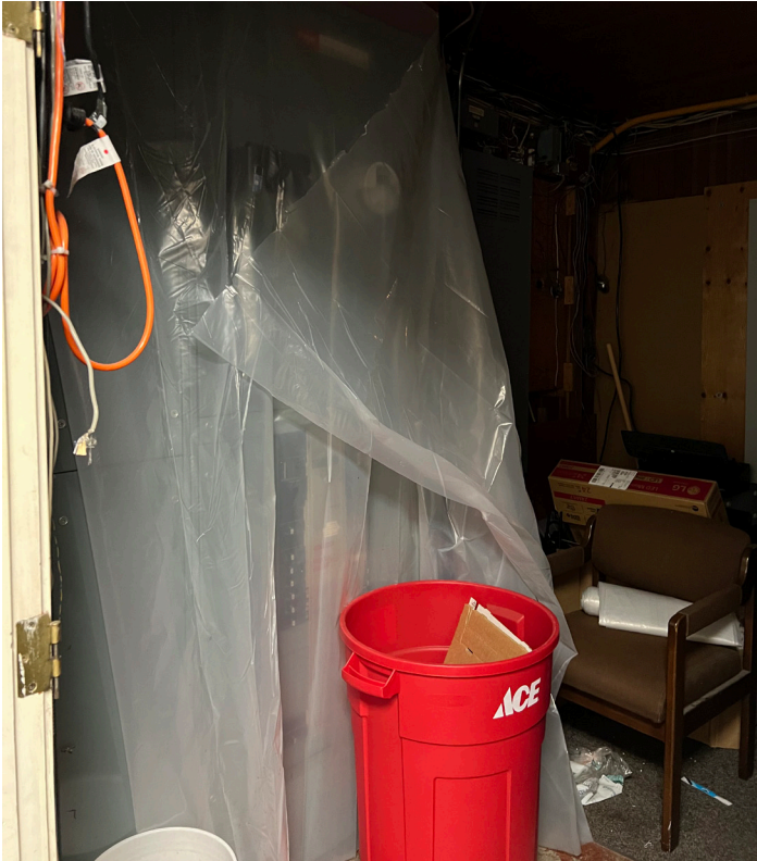
Switchboard Protected from Water - Police Station
