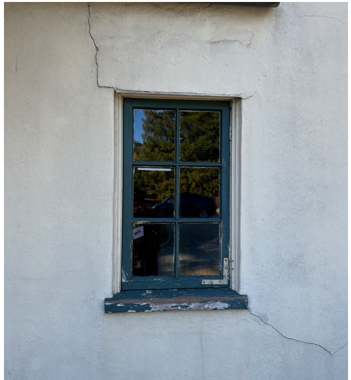
Public Safety Building - Deteriorated Exterior Enveloped
