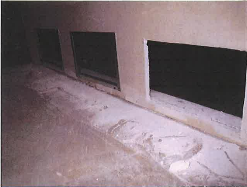
View of flood ports: in the garage at 81 Sir Francis Drake Blvd., Ross, CA 94957. Photo taken December 1, 2009.
