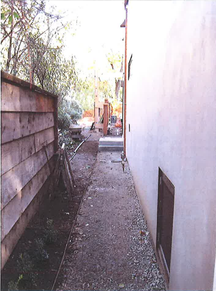
View of flood port: North side of 81 Sir Francis Drake Blvd., Ross, CA 94957. Photo taken on November 15, 2009.
