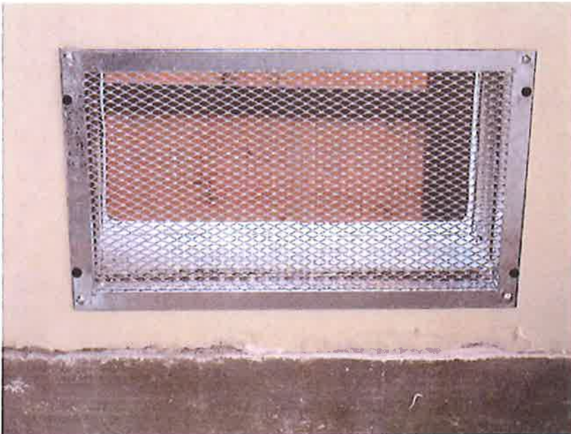
View of flood port: on North side of garage at 81 Sir Francis Drake Blvd., Ross, CA. Photo taken on December 1, 2009.
