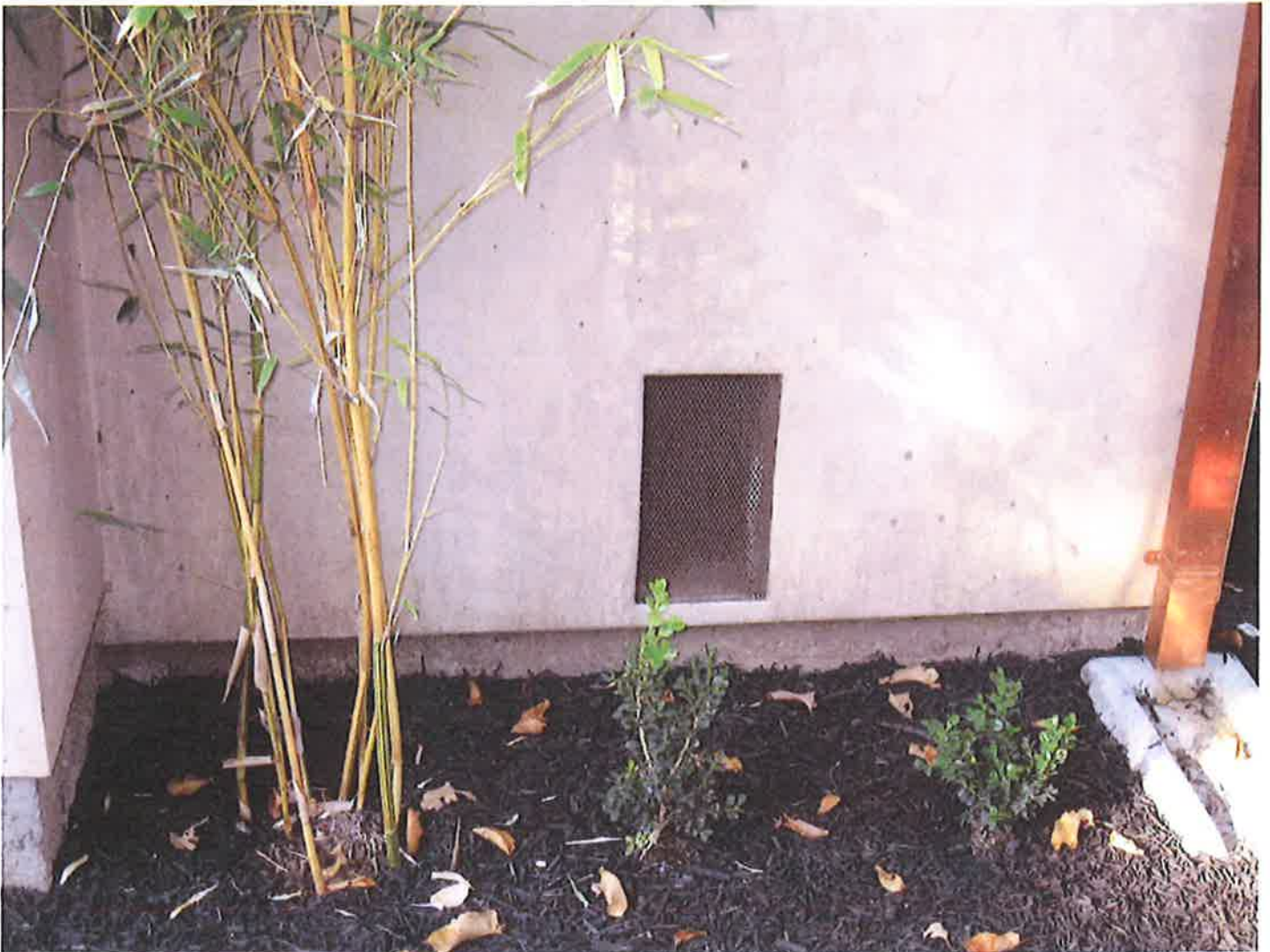
View of flood port: South side of 81 Sir Francis Drake Blvd., Ross, CA. Photo taken on November 15, 2009
