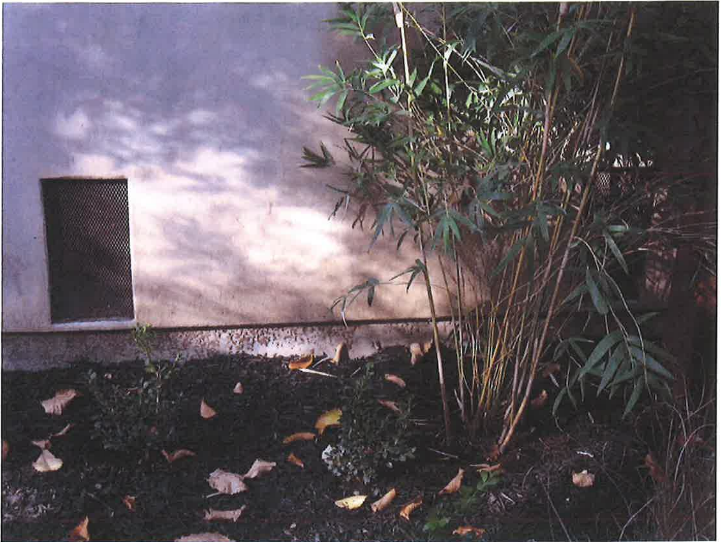
View of flood ports: South side of 81 Sir Francis Drake Blvd., Ross, CA. Photo taken on November 15, 2009.
