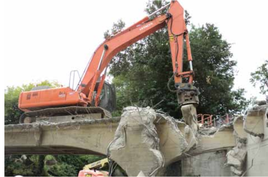
The Town awarded the Lagunitas Road Bridge reconstruction contract and demolition work began shortly thereafter.
