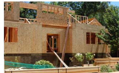
This house on Sylvan Lane is being raised above the 100-year flood level.
