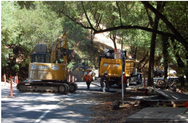
Culvert repair work on Laurel Grove Avenue, one of the public works projects funded in the 2011-2012 budget.
